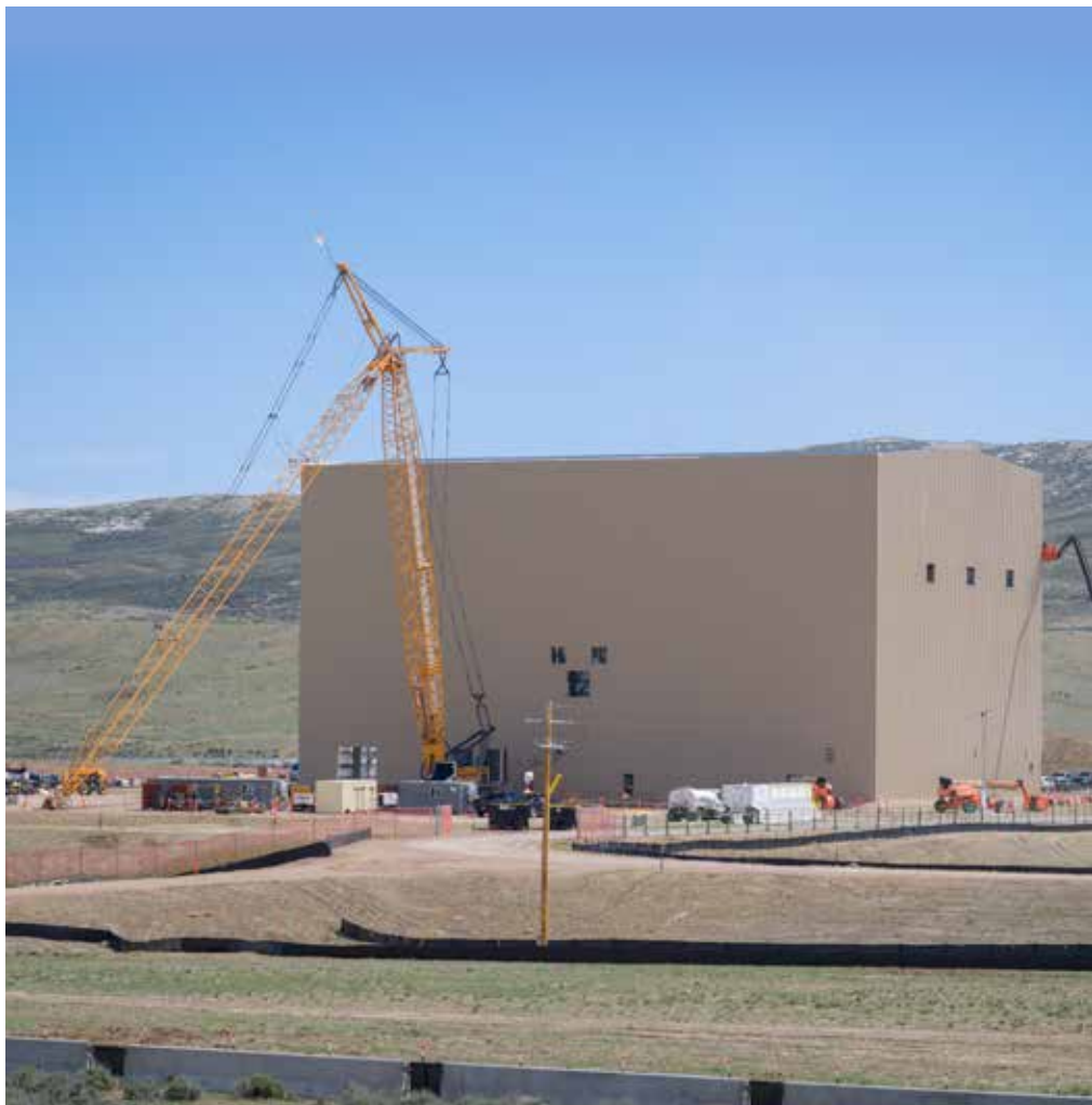
Construction of the TerraPower nuclear reactor is underway in Kemmerer, Wyoming (May 27, 2026). The reactor, which is expected to begin generating power by 2031, will support data centers and the artificial intelligence boom.
